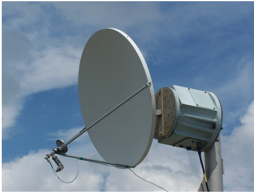
Figure 2: Antenna mounted for test
